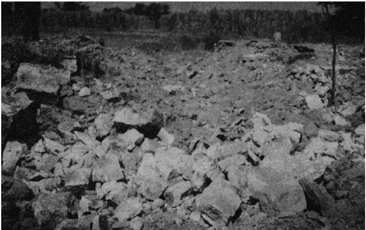
Culvert on Annaran-Reddipet blasted by Naxalites by claymore mines
